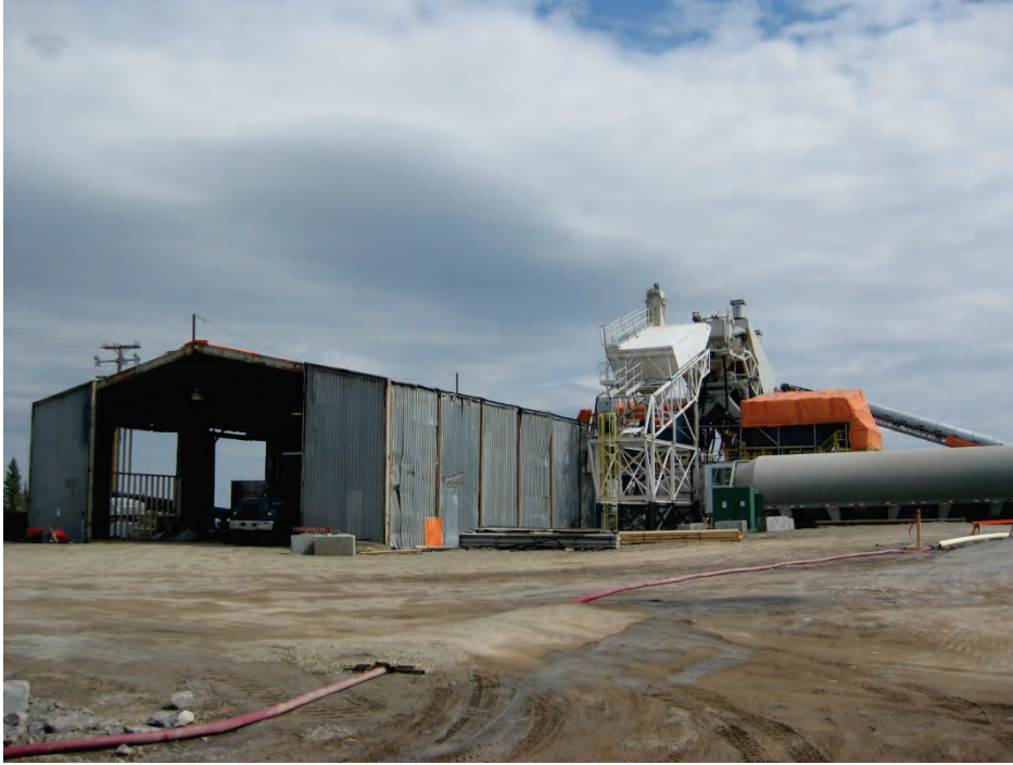
Photograph 3-2: Typical Concrete Batch Plant (Wuskwatim Project, Manitoba Hydro, 2009)
