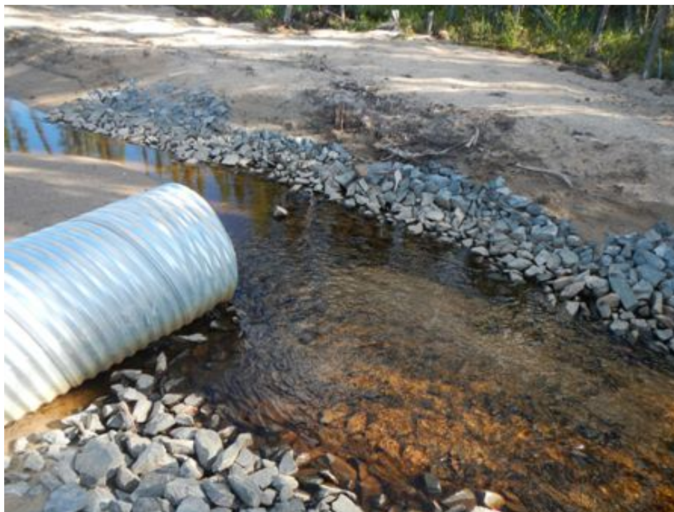
Figure 4. Unnamed tributary flowing through the culvert during construction – rip rap placed to control erosion of material.
