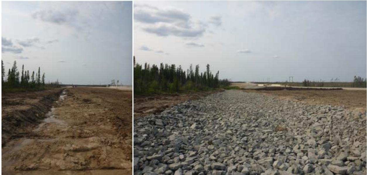
Figure 3: Erosion control measures installed along road embankment near Looking Back Creek, before and after photos
