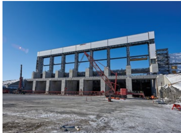
Downstream view of the Spillway. Main gates are now fully installed; gate and hoist work continues to support river diversion targeted July.
