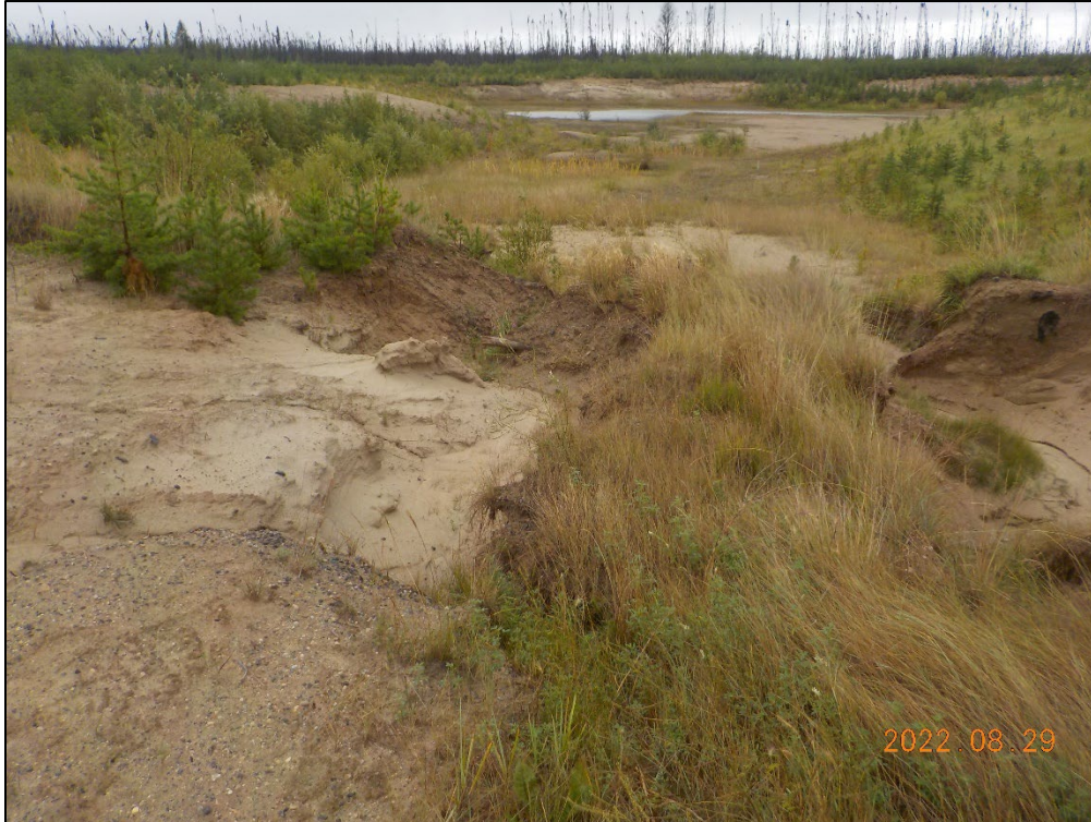
Photo 3-11: Erosion and affected planted seedlings in Borrow Area KM-1 in 2022
