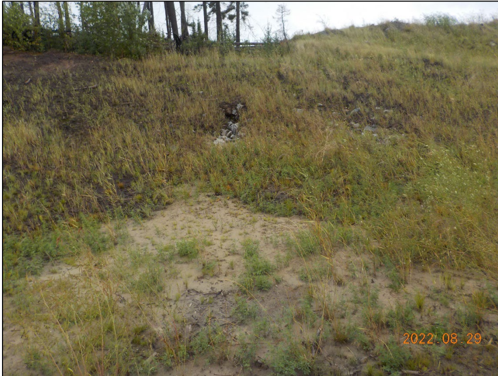
Photo 3-2: Erosion on NAR side bank adjacent to Borrow Area KM-1 in 2022
