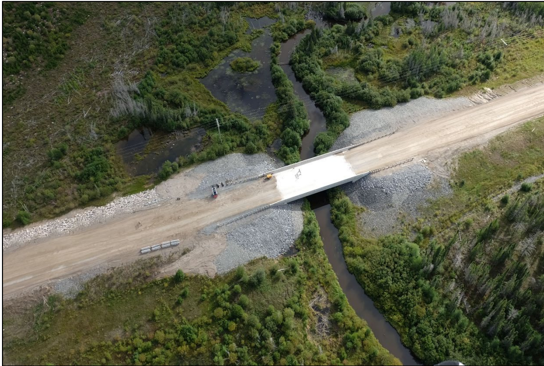
Photo 3-3: Construction work on the North Access Road adjacent to Looking Back Creek in 2022
