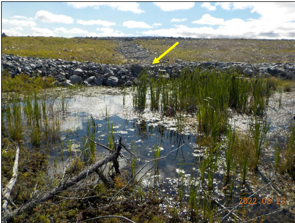
Photo 3-4: Filled gap in rock berm (yellow arrow) and ponding water in the Wetland 51 buffer zone.
