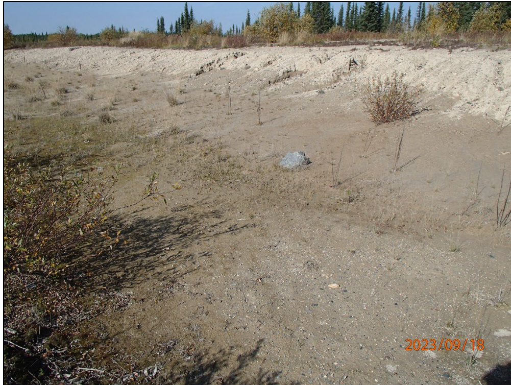
Photo 4-13: Barren, eroding slope along the South Access Road in 2023
