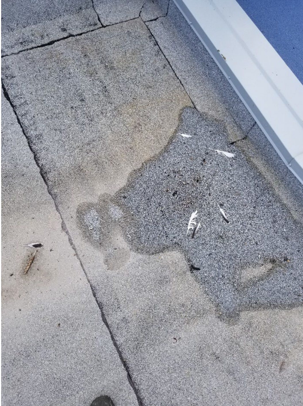
Photo 3: Feathers and Fish Spine on Powerhouse Roof, July 2023
