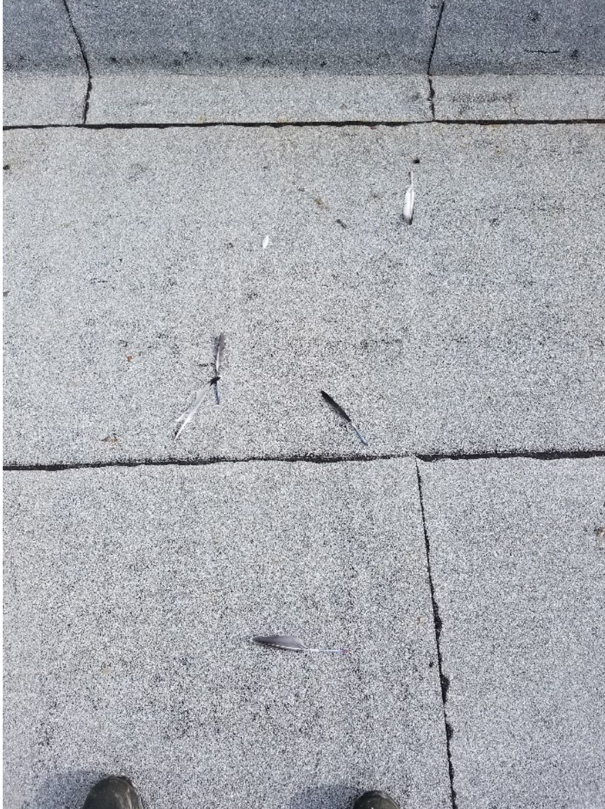
Photo 2: Feathers on Powerhouse Roof, July 2023
