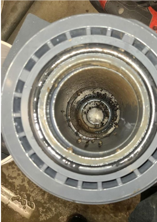
Figure 7: Example of zebra mussels growing inside a water pipe.
